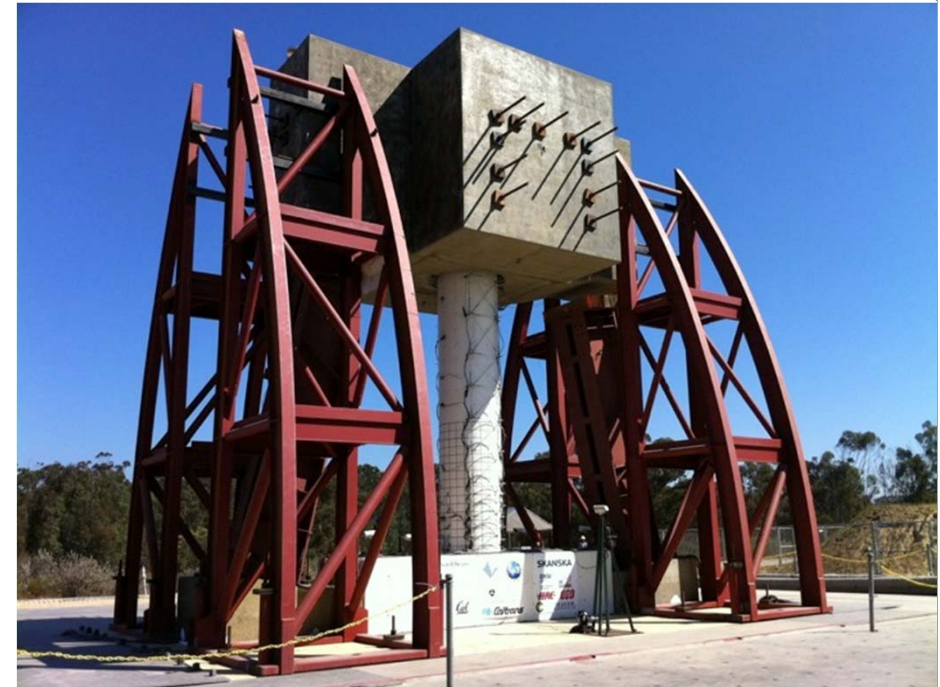
Full-scale 1D tests of circular column - Jose Restrepo, PI (PEER, Caltrans, UNR, FHWA, NEES@UCSD, NEEScomm & NSF)
