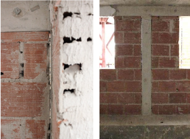
Separation between frame and infill
