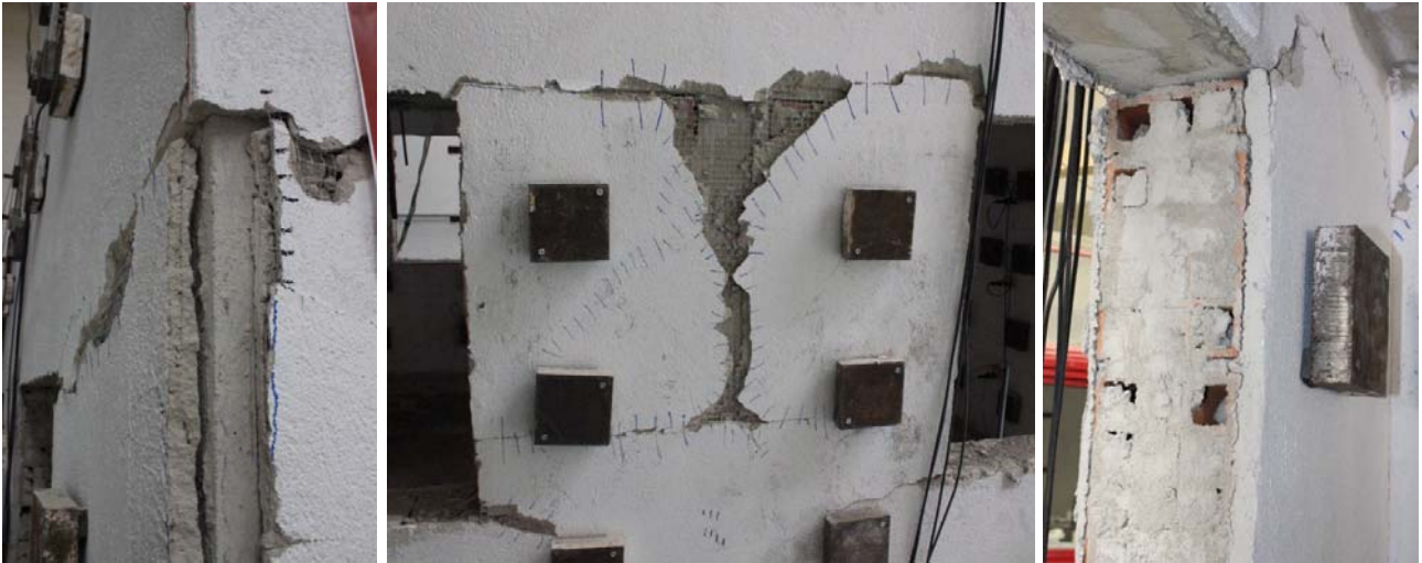
Cracking in rendering around openings and corners
